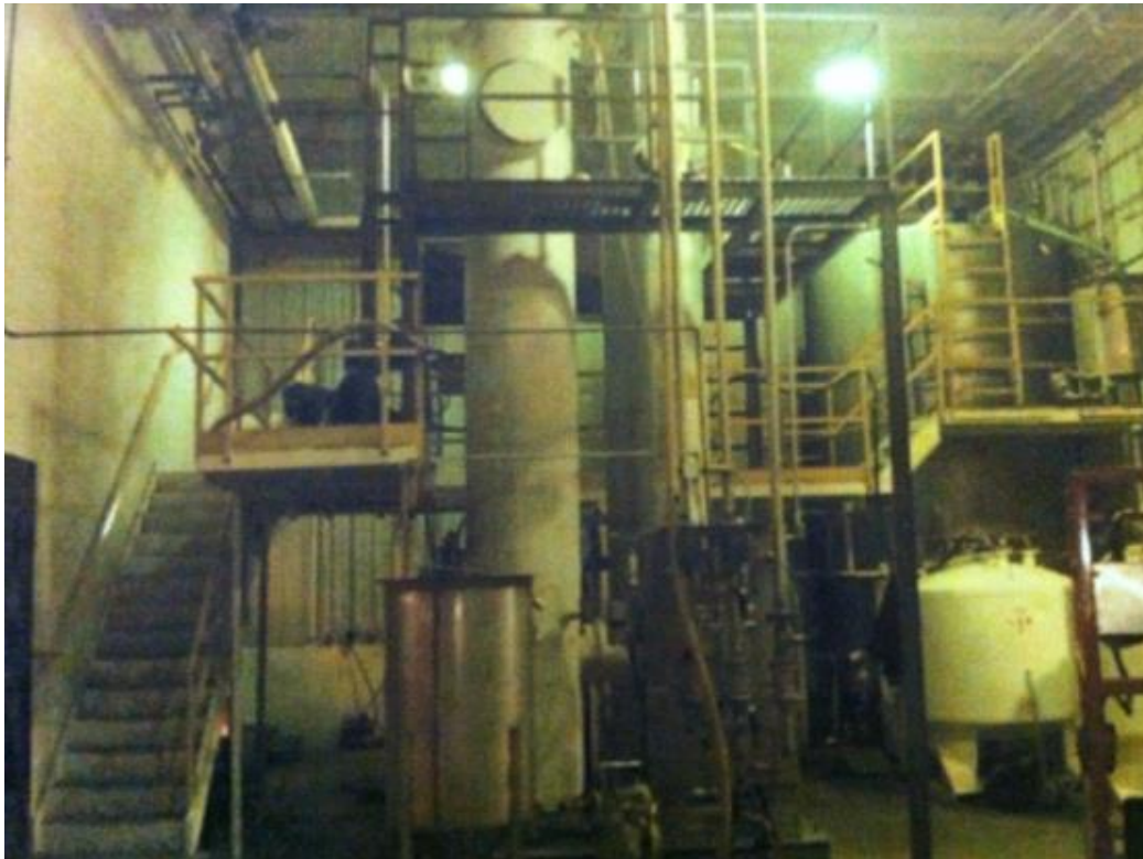
Two ammonia strippers are shown in the center of the picture
